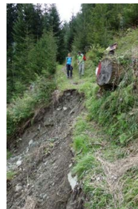
Figure 1: Landslide damage on hiking trail
