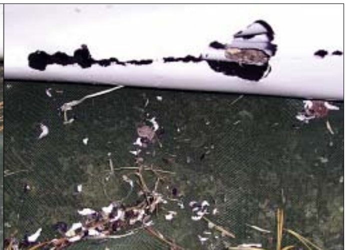
Figure 4: Mice damages on the plastic film and the original mouse protective grid
